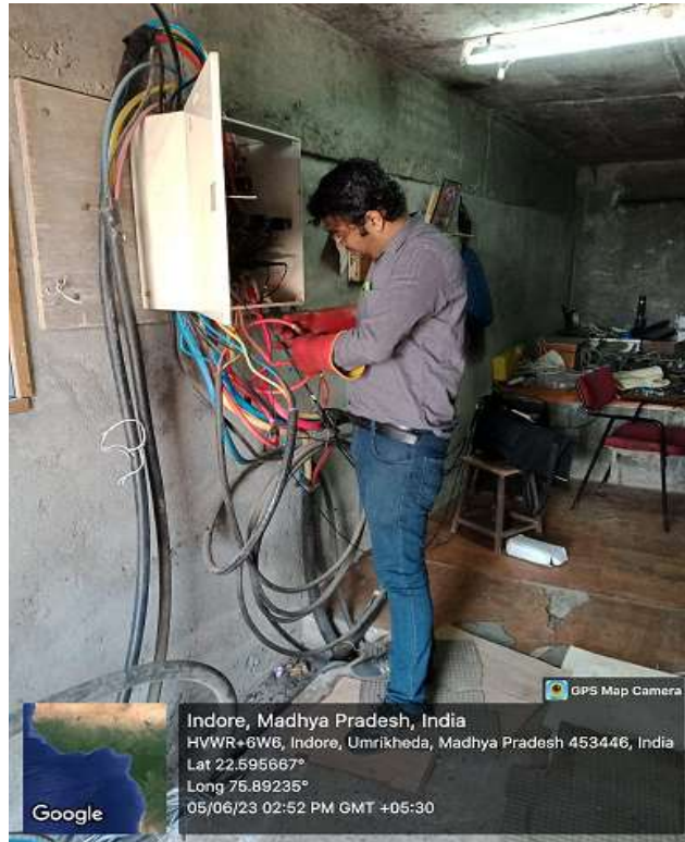
Fig. 4.2- 24 Hours 3-phase load recording by power analyzer LM-30
