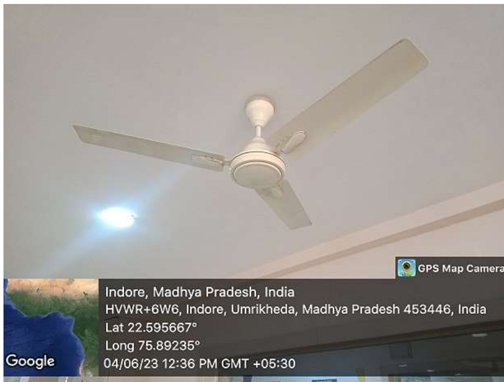
Figure 4.4 Electrical Equipments in college
