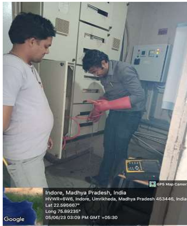
Fig. 4.3- Engg. Block 3-phase load recording by power analyzer LM-30
