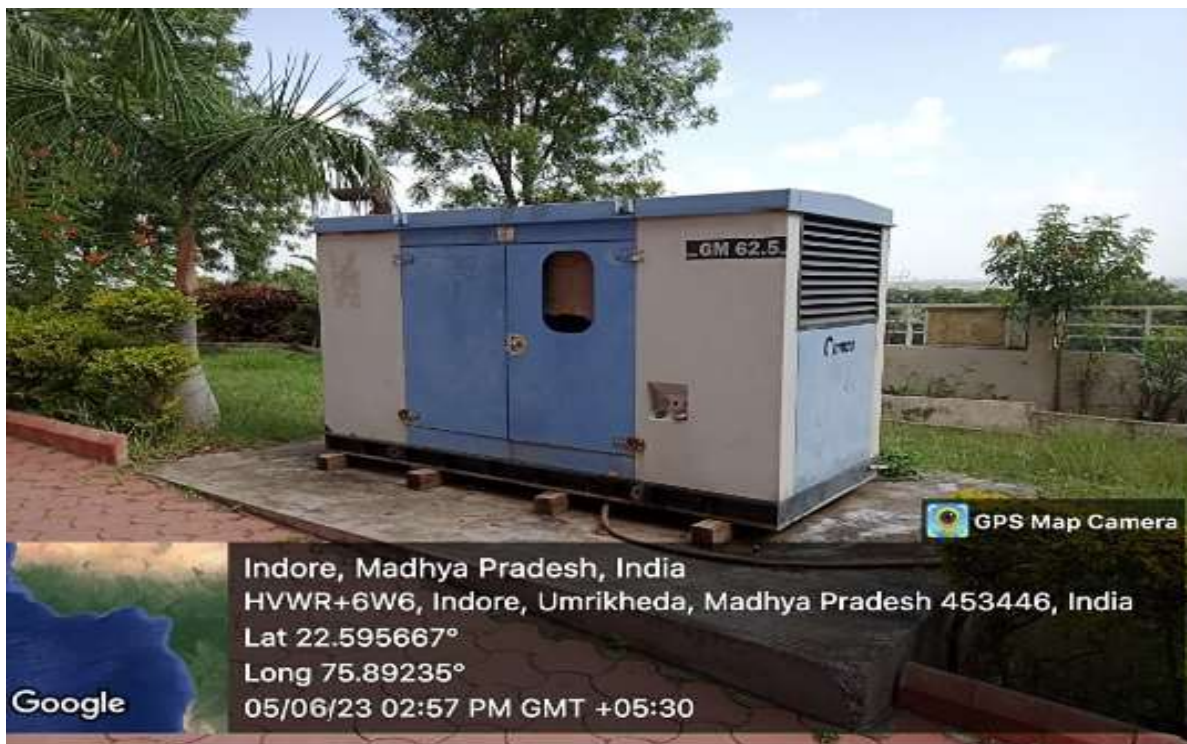
Figure 2.3:- DG set in the campus
